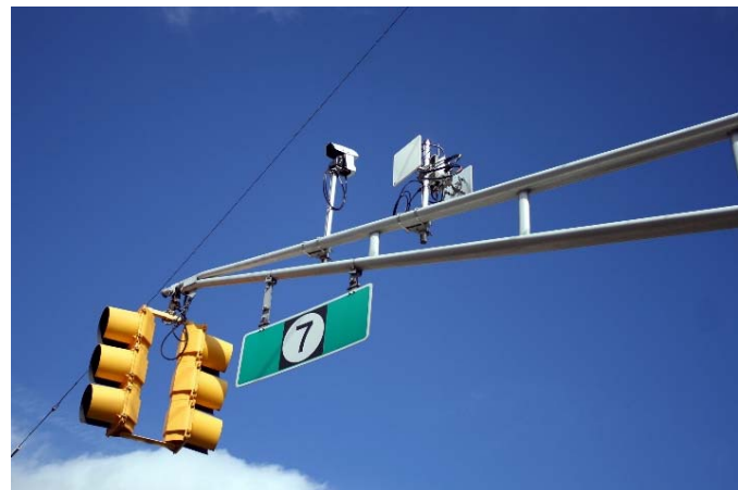
Figure 41: Adaptive Signal detection camera and radio on a traffic signal mast arm (Source:
