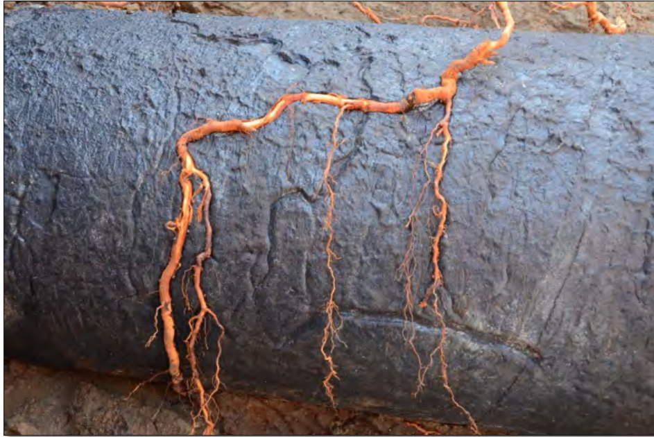
Figure 24. At dig site RWVIM-165-13 some impressions still had roots imbedded while other impressions were vacant.
