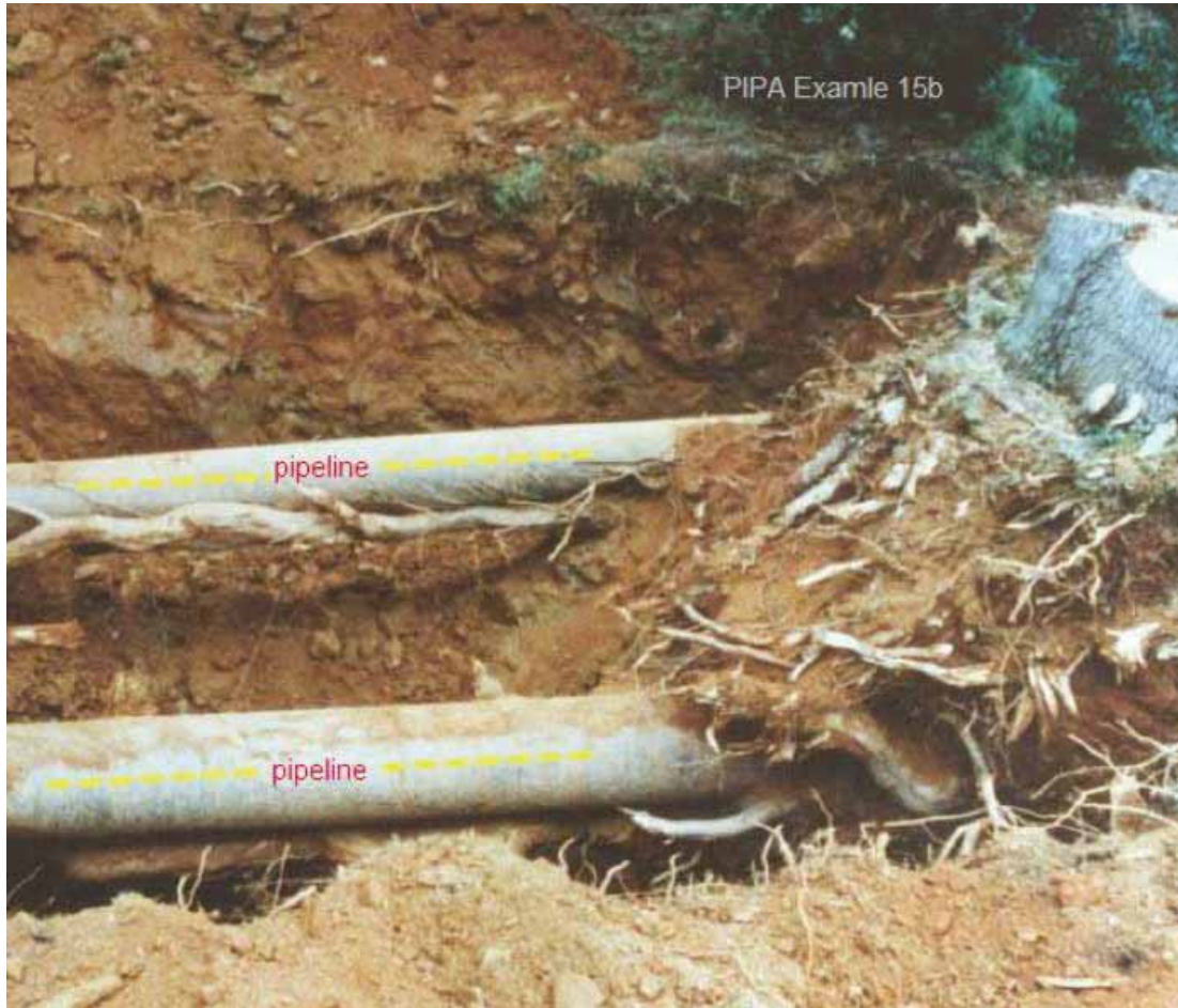
Figure 4. Roots in proximity to buried utility lines (note proximity of trunk to pipes). Pipe diameter is unknown, but appears to be approximately 6 inches. Photo from PIPA (2010).
