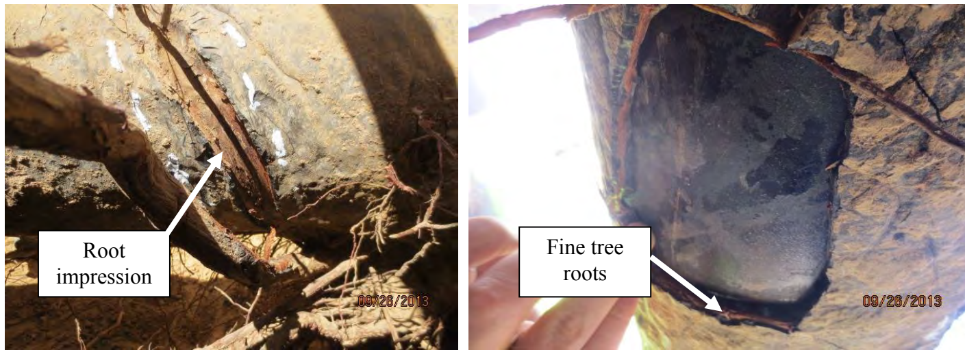
Figure 4. Photographs from Dig RWVIM 76-13 showing: A root impression in the coal tar enamel coating (Left) and disbonded coating with root intrusions (Right).
