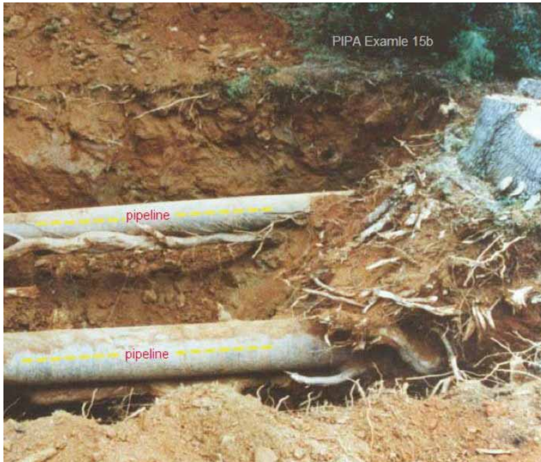
Figure 4. Roots in proximity to buried utility lines (note proximity of trunk to pipes). Pipe diameter is unknown, but appears to be approximately 6 inches. Photo from PIPA (2010).
