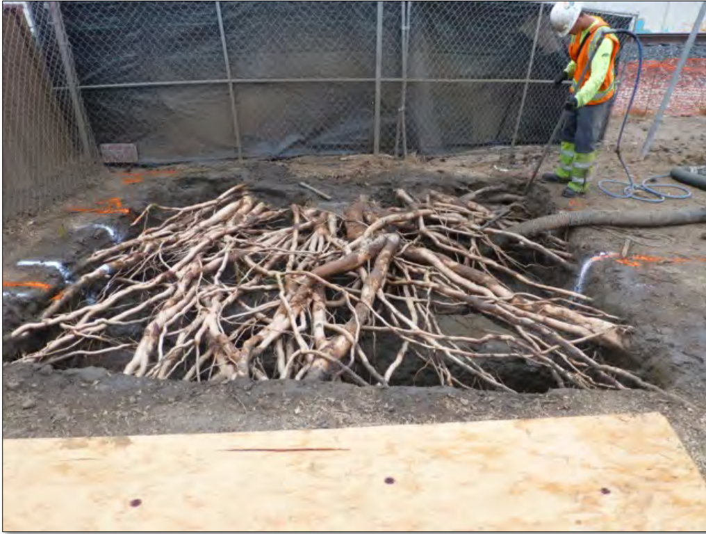
Figure 2. The hydro-vac process uses high pressure water and a large suction hose to excavate soil leaving the roots intact.
