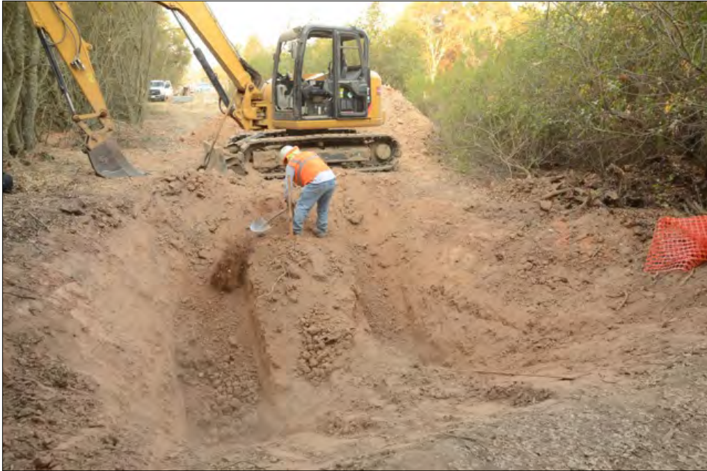
Figure 3. This is a dry dig site using track hoe and shovels to excavate soil and roots.
