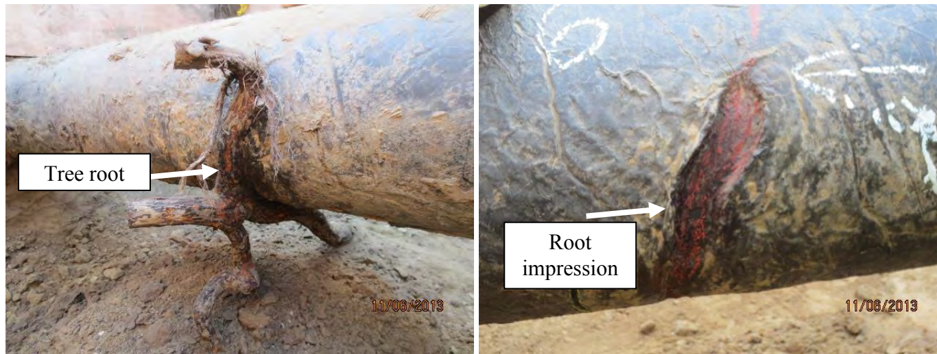
Figure 3. Photographs showing the interaction of a tree root with the pipe section from Dig RWVIM-259-13, which was coated with hot applied asphalt: Tree root in contact with pipe (Left) and coating damage after the tree root was removed (Right).
