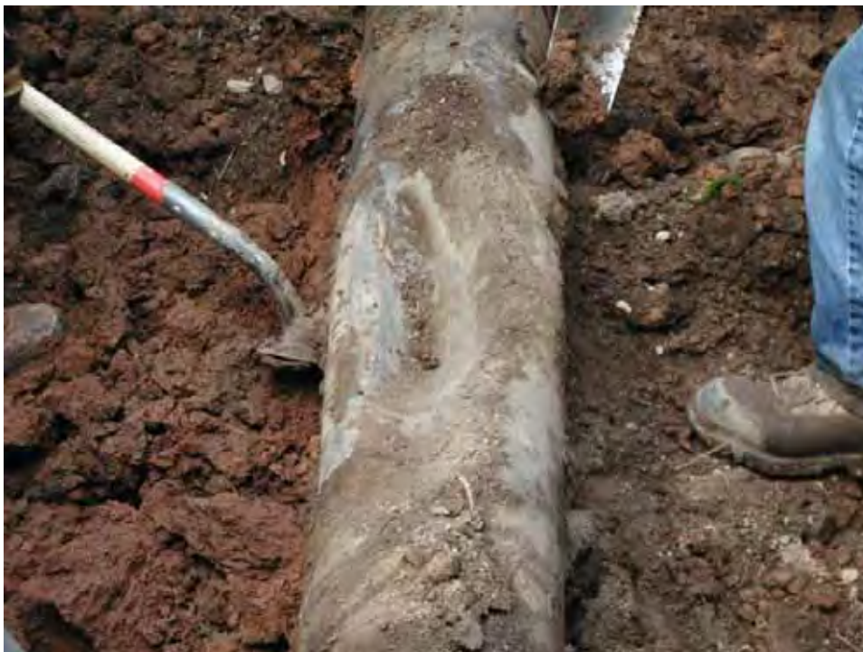
Figure 13. Apparently, the top of this pipe was dented by the explosive expansion of soil after a tree was struck by lightning, as described in Figure 12. Photo from PIPA (2010).
