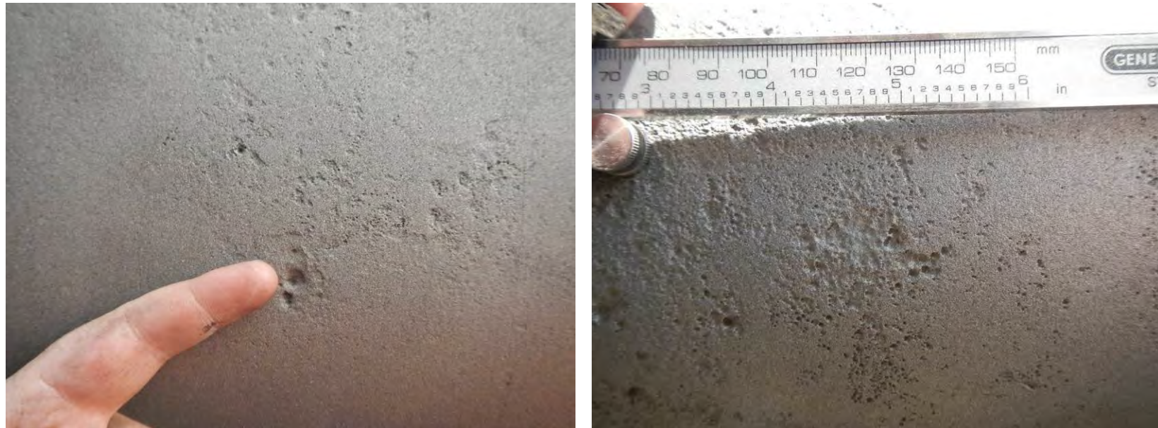
Figure 7. Representative photographs showing external corrosion on pipe segments.
