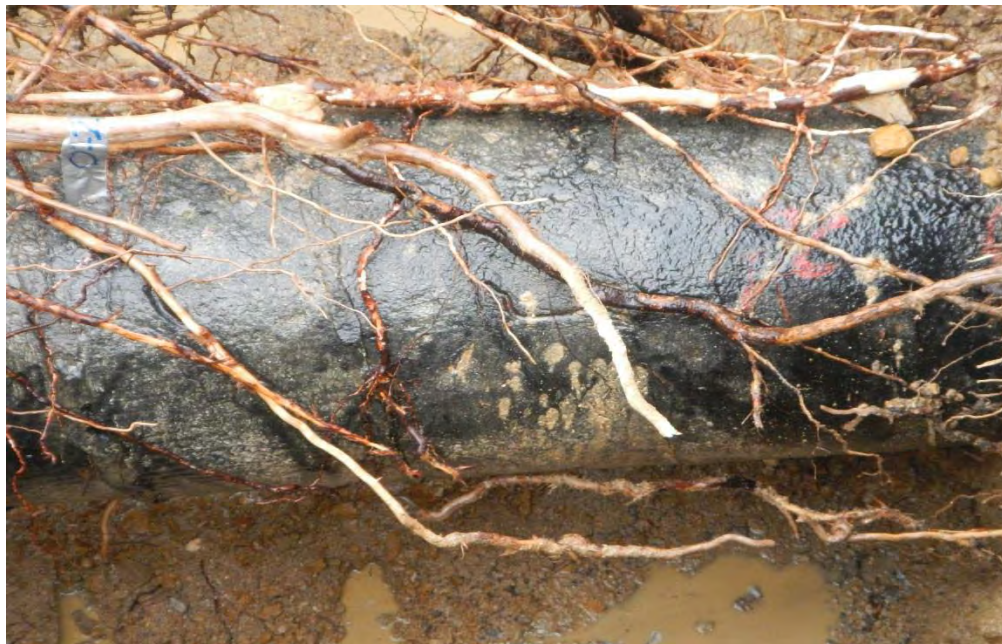
Figure 4. RWVIM-74-13 (Atascadero) (HAA coating damage)
