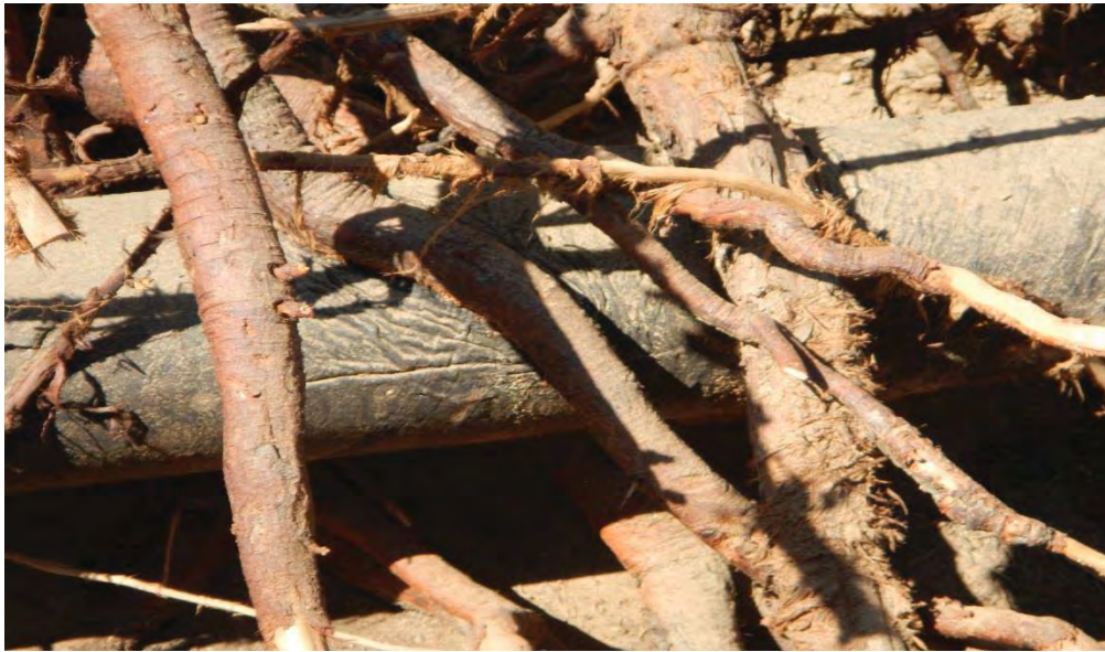
Figure 3. RWVIM-107-13 (Weber Lane) (CTE coating damage)
