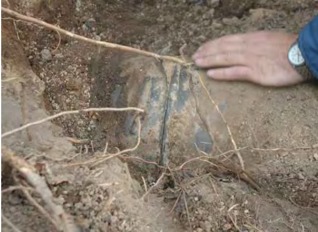
Figure 14. Tension in the pipeline caused by the lightning strike described in Figure 13 resulted in the formation of a crack in a girth weld in the pipe. Photo from PIPA (2010).
