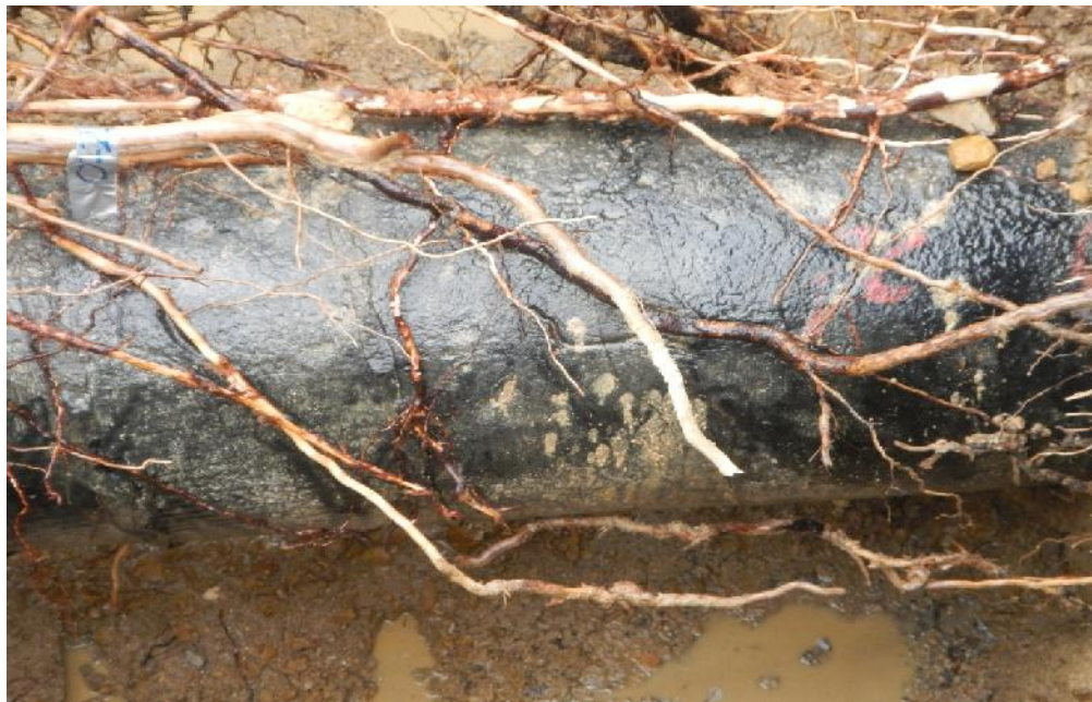
Figure 4. RWVIM-74-13 (Atascadero) (Tape coating damage)
