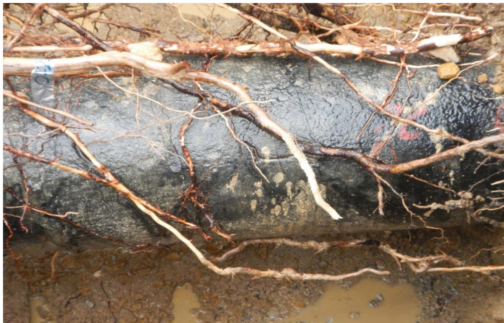
Figure 4. RWVIM-74-13 (Atascadero) (Tape coating damage)
