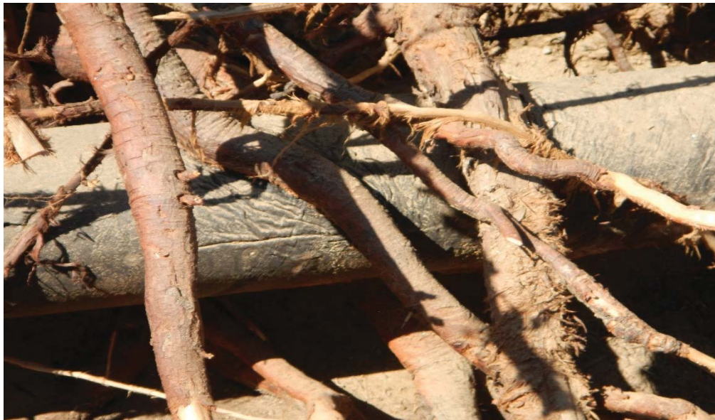
Figure 3. RWVIM-107-13 (Weber Lane) (CTE coating damage)
