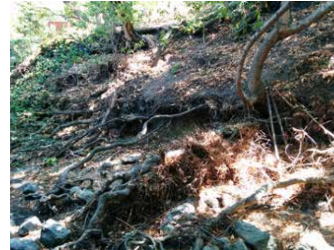
Undercutting of bank
