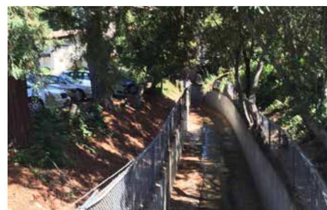
Creek channel velocity is dangerous during rain events.
