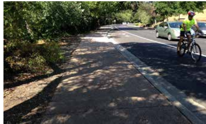
Pervious paving would connect to sidewalk segment directly to the west of this reach
