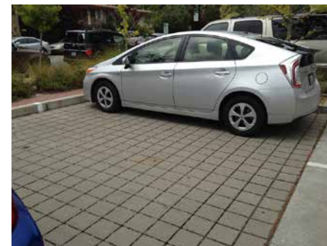
Pervious pavers in parking lot
