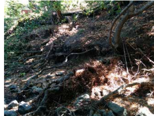
Undercutting of bank
