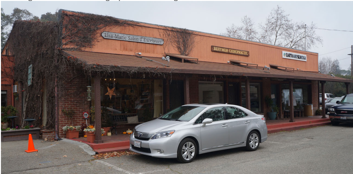
View of the south wall of the east side of Building 2, the first section at 3674-78 Mt. Diablo Boulevard.
