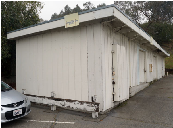
View showing the south (left) and east (right) walls of the storage building (Structure 2).
