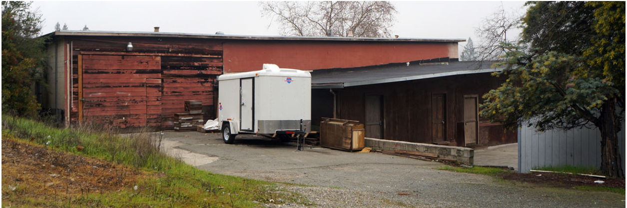
View of the north side of the west exterior wall of Building 1, looking east.
