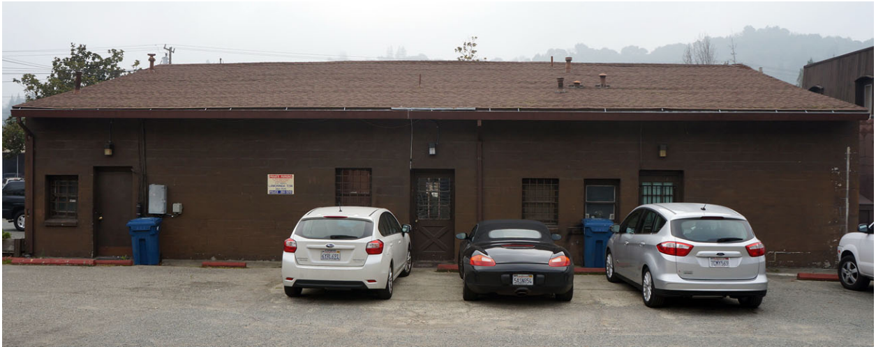
View of the north or rear exterior wall of the first section of Building 1 at 3674-78 Mt. Diablo Boulevard.
