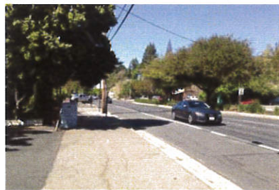
6. Existing street frontage and broken sidewalk
