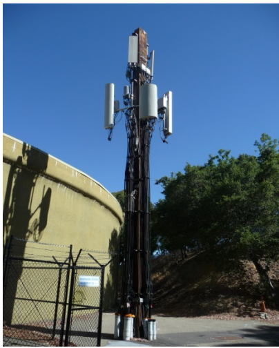
1) End of Kim Road 167-040-018 AT&T
