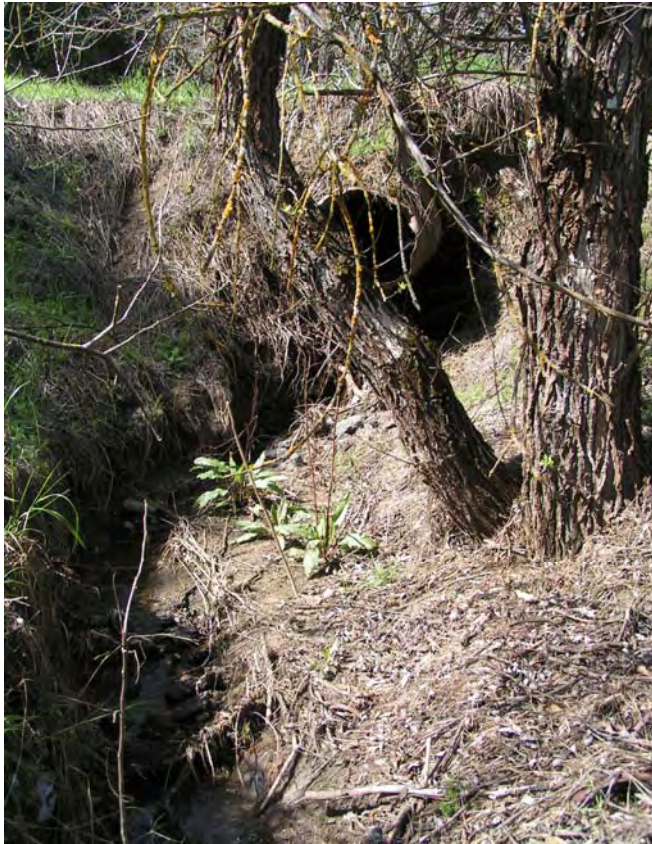
Photograph 5. Old defunct metal culvert spanning channel of drainage, facing northwest. High-flows have blown-out the downstream portion of the drainage in this reach, and waters have undercut the channel bed beneath, bypassing the culvert.
