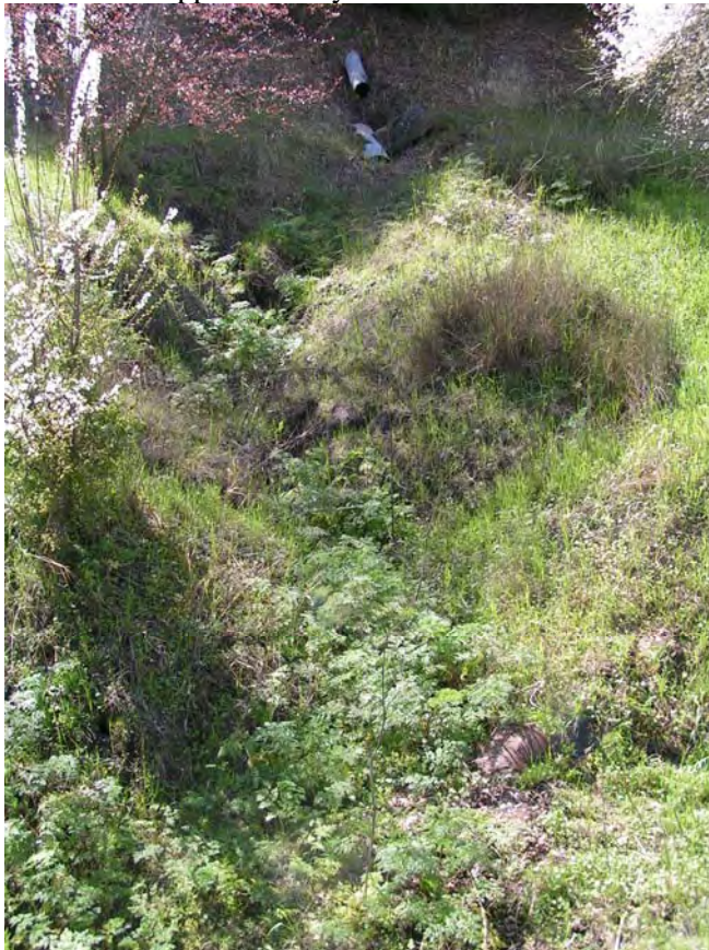
Photograph 4. Drainage created by scour conveyed by metal culvert (in top of frame) underneath blacktop driveway that intercepts runoff from the western portion of the Property.
