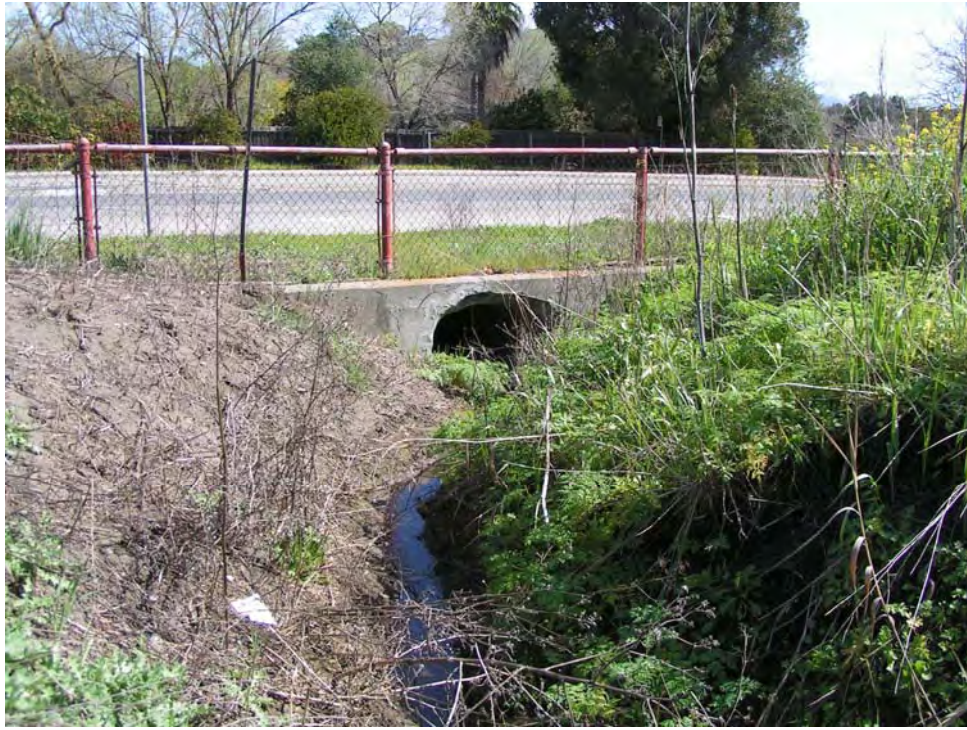
Photograph 1. Concrete culvert underneath Pleasant Hill Road along the eastern boundary of the Property, facing southeast. This feature is a tributary of Reliez Creek, located approximately 0.25-mile east.
